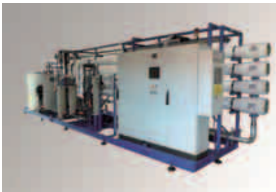
PVS RO Plant
